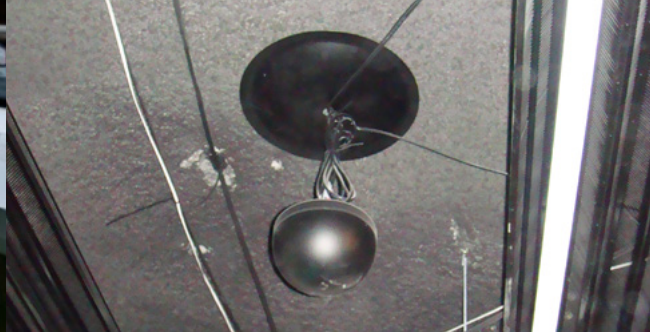
Installed transducer with acoustic disc
