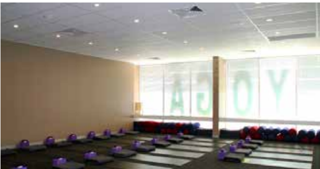
The glass walls and thin ceiling allowed intrusive noise to impact the comfort of the occupants
