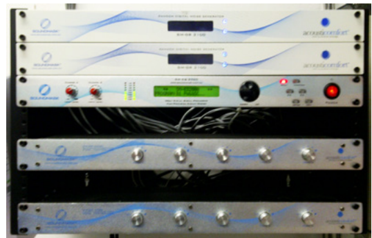
Soundmask system components neatly secured on a rack unit
